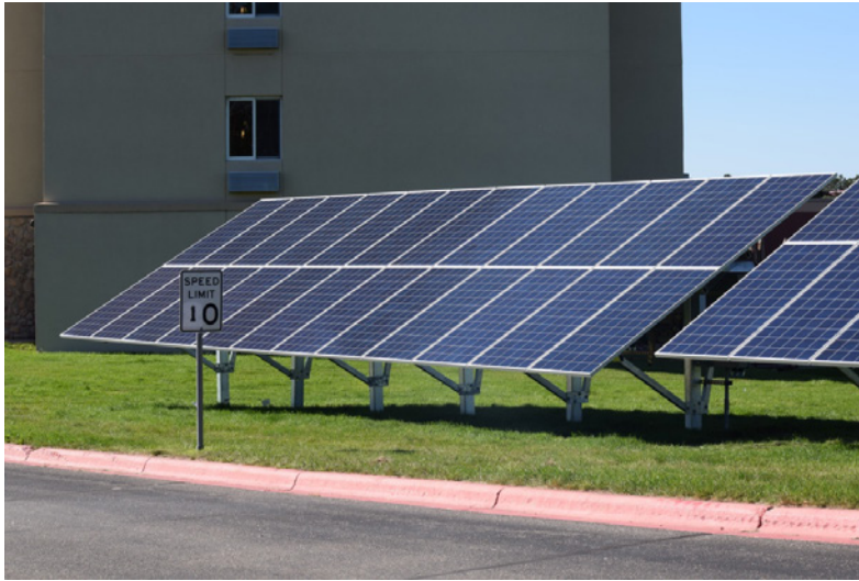
New solar panels were installed at the Northern Lights Casino and the Leech Lake Band of Ojibwe Administration building in September.
