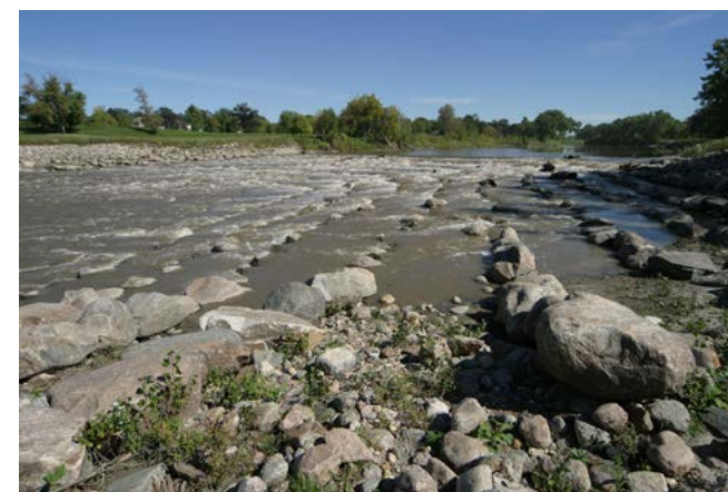
Red River of the North rock structure located in Grand Forks. This photo is taken from the river bank looking upstream towards the dam. There was about five feet of head on this dam.
