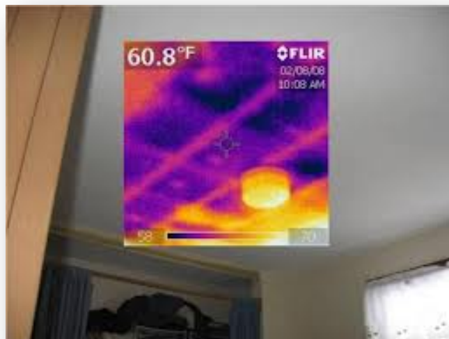
Booth Bay Register/Thermal imaging
